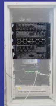
1/2 Rack BBU Servers
